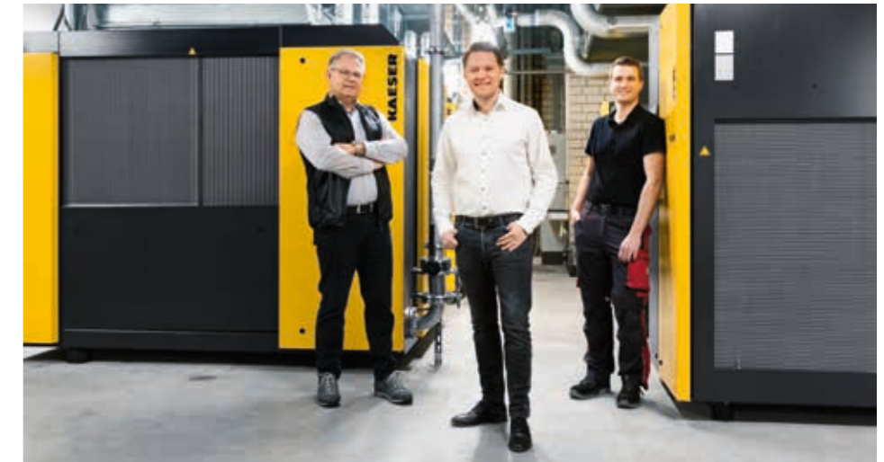
Managing Director Florian Müller-Stauch (centre), Head of Plant Engineering Dirk Brinkmann (left), and Deputy Head of Plant Engineering Yannic Ostermann (right) are delighted with the new compressed air station from KAESER.
