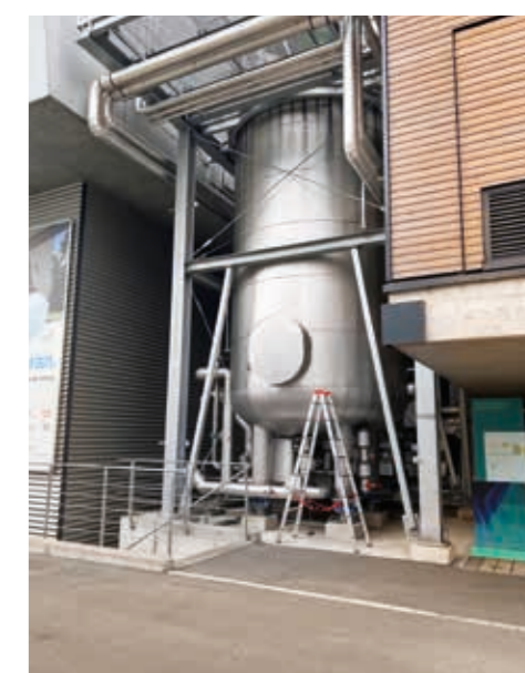
The heart of the power-to-gas plant: the bioreactor.
